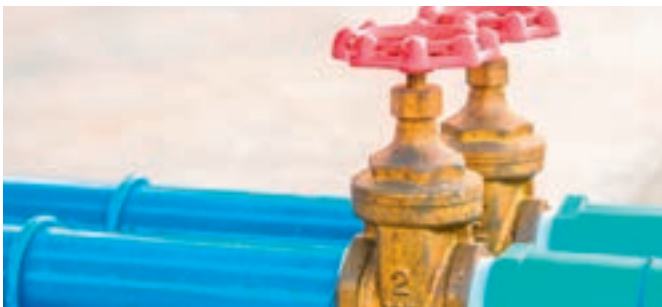
Fittings/valves, also oxygen-supplying
